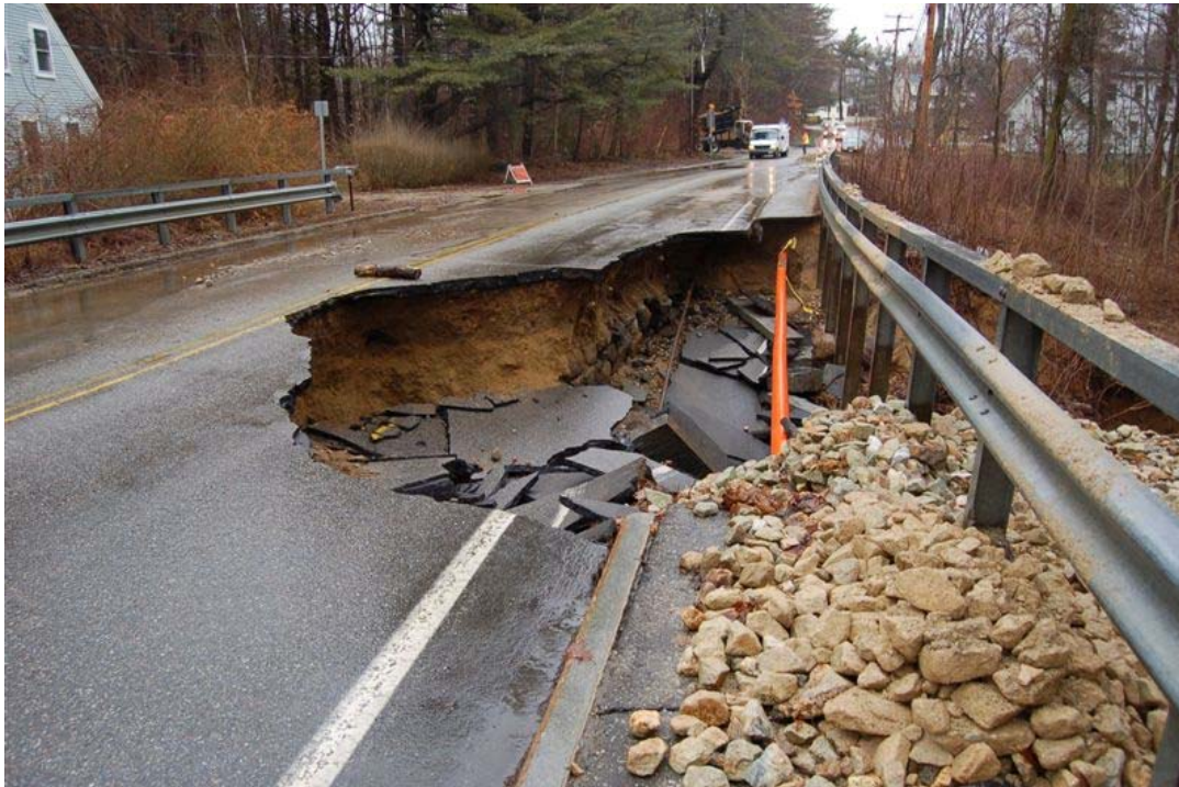
Figure 6.4 An example of unexpected severe erosion caused by flooding in Dover, New Hampshire, April 2007. 208
